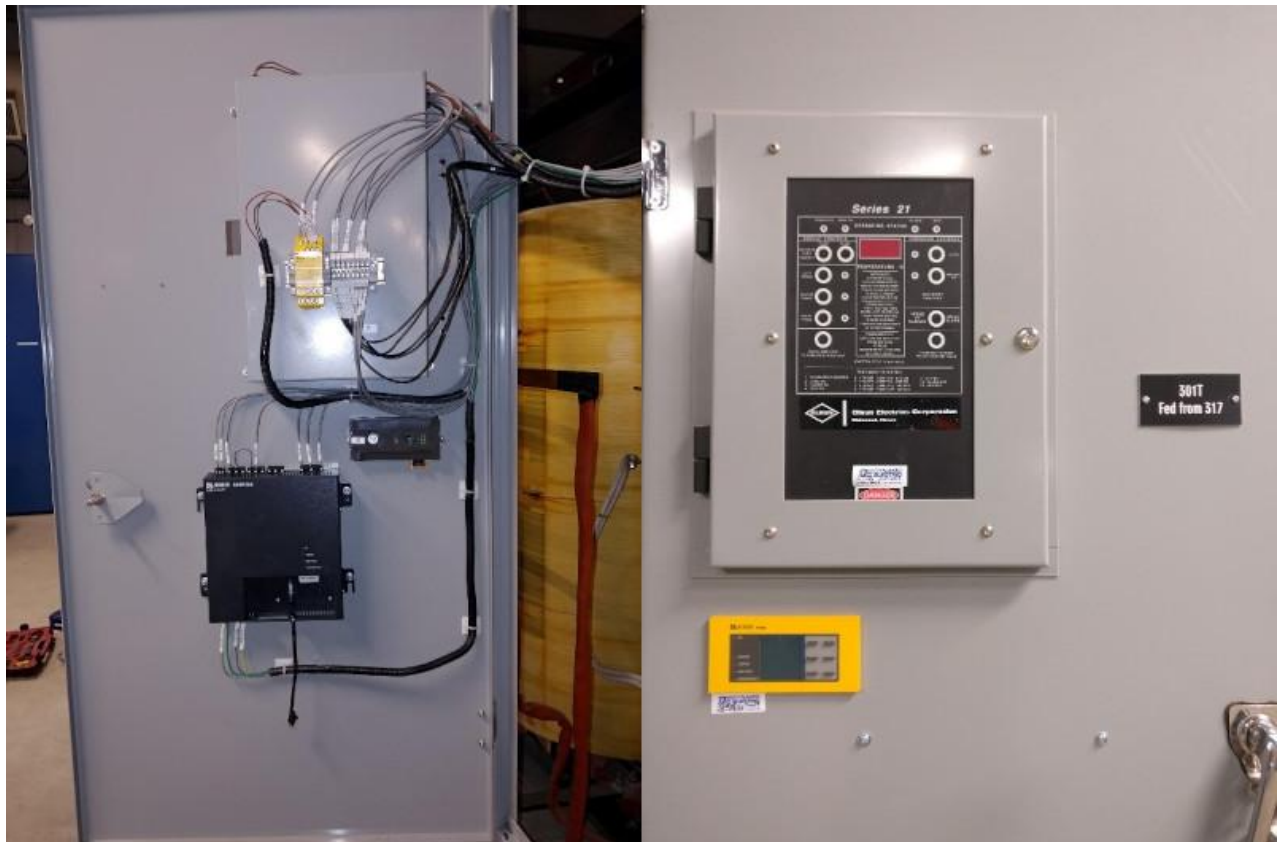
Image 1: NGR monitor components installed on back and front of transformer section door.
