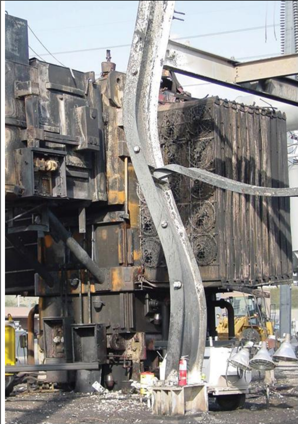
Remnants of a large transformer fire
