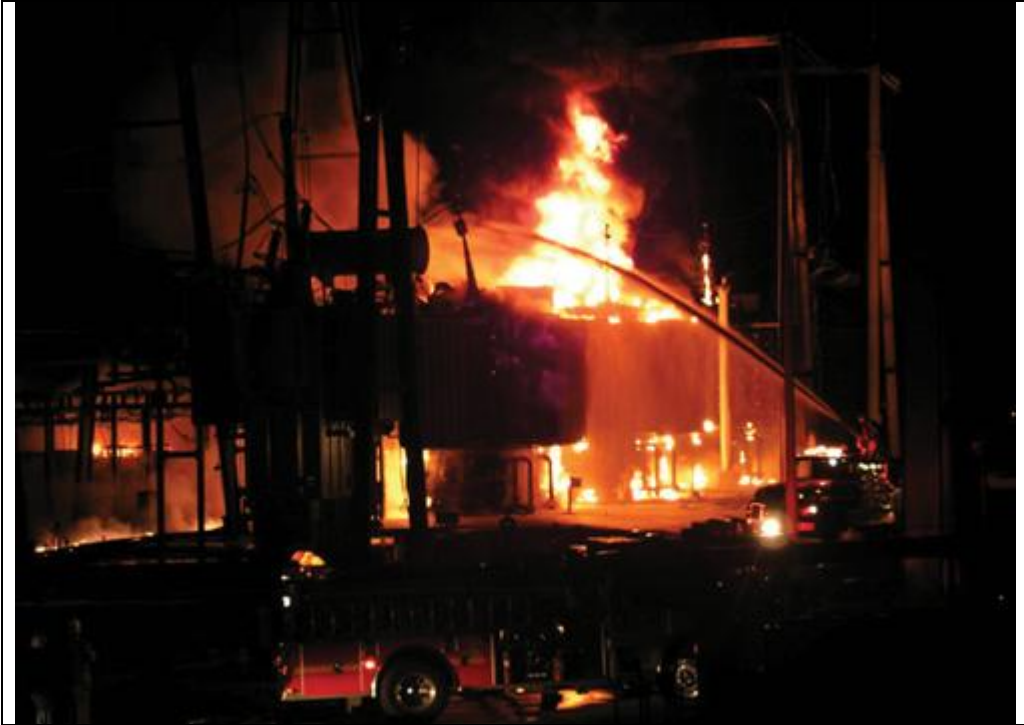
Initial transformer fire ignites neighboring transformer
